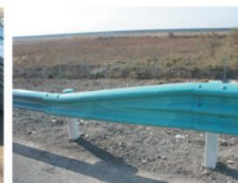
◎二变三护栏/ Two to Three Wave Guardrail
